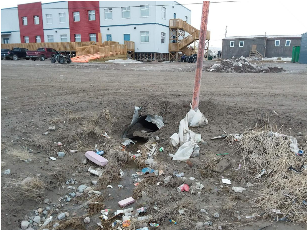
Figure 38: End of blocked culvert looking west from side of 6 th street
