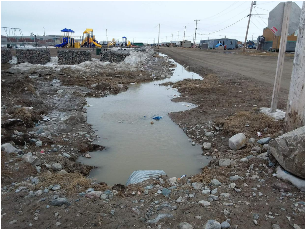
Figure 6: Condition of ditch on northwest side of 7 th Street at 9 th Avenue intersection
