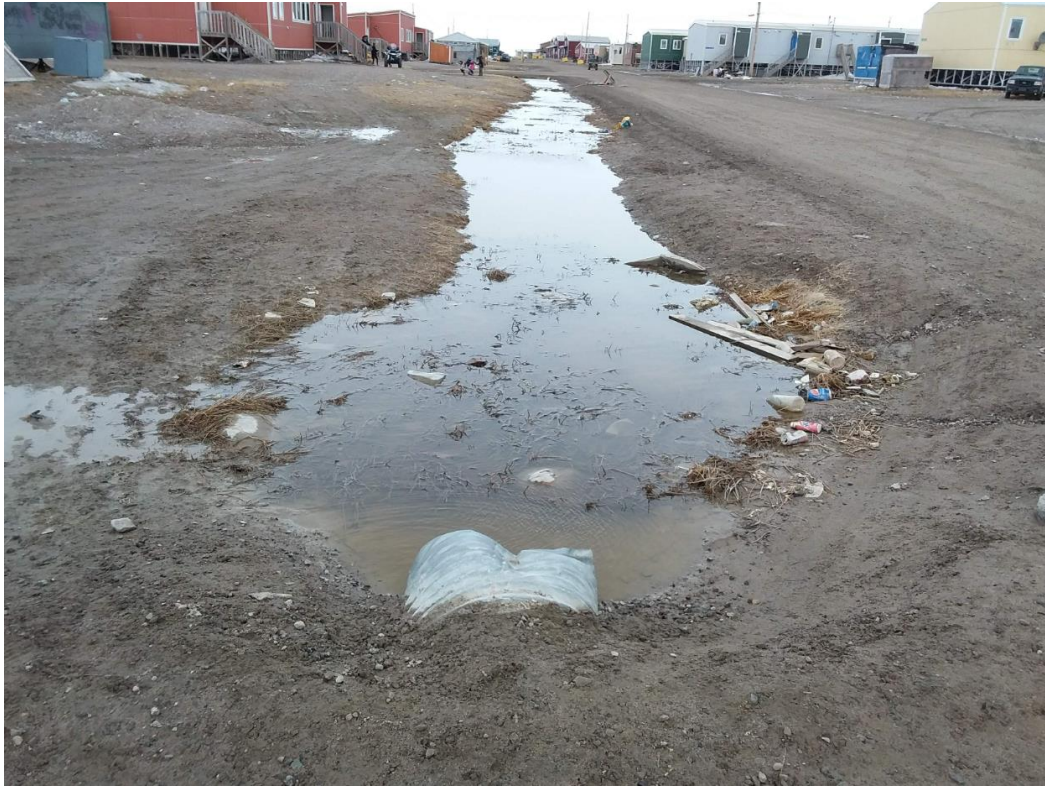
Figure 4: Condition of ditch on northwest side of 8 th Street at 9 th avenue intersection
