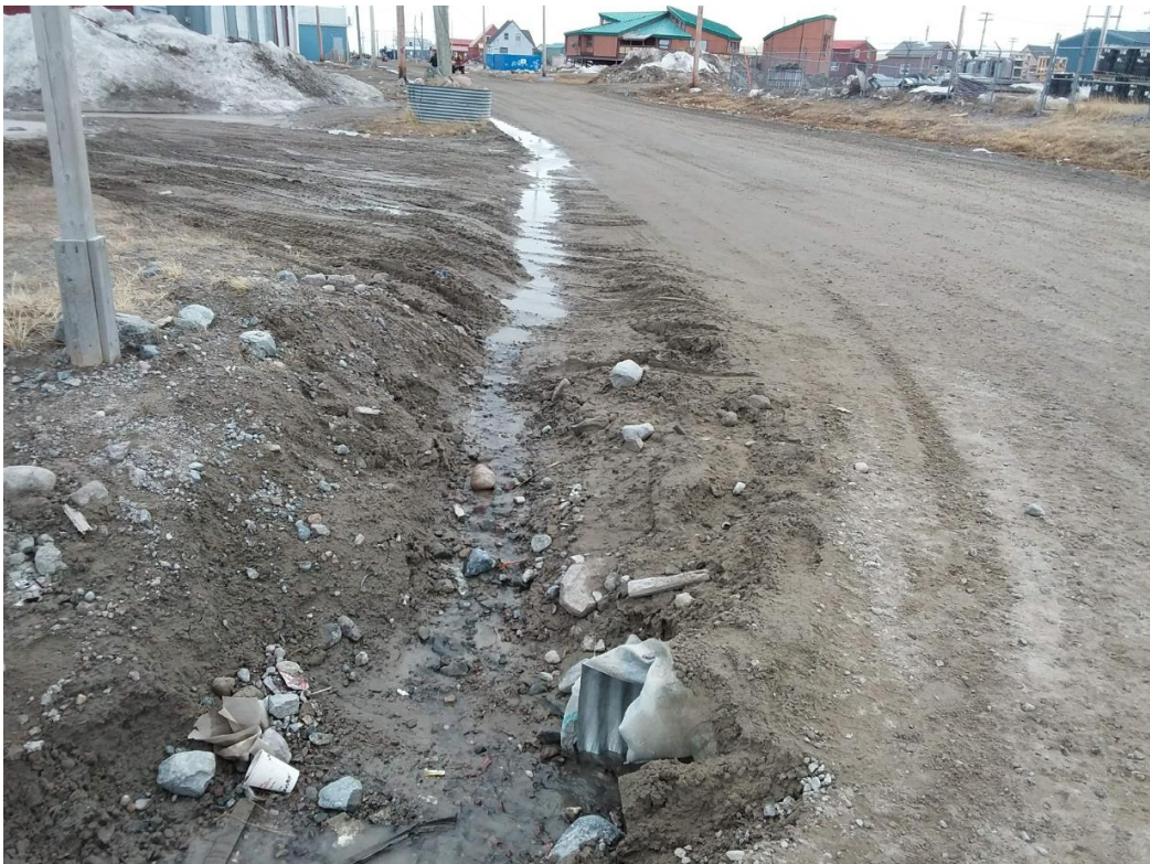
Figure 22: Ditch condition on west side of 6 th street near 4 th avenue
