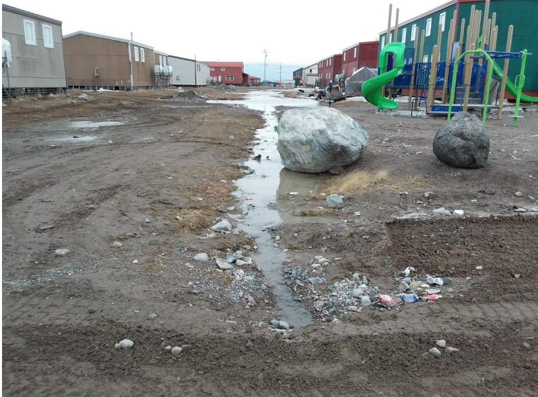
Figure 35: Looking east between properties at end of culvert off of 4 th street
