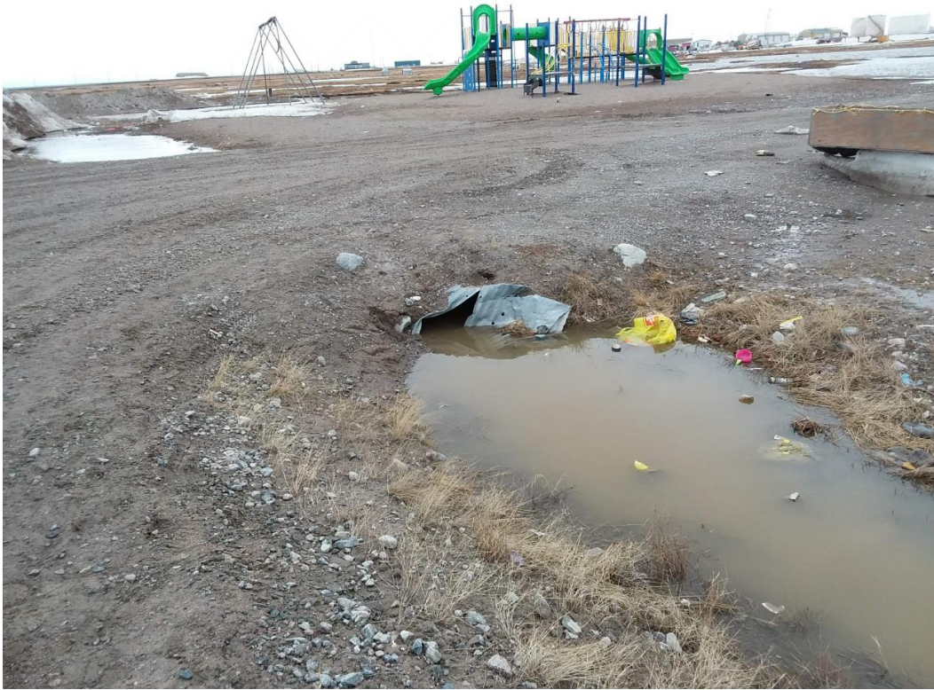
Figure 3: Blocked culvert at playground looking southwest
