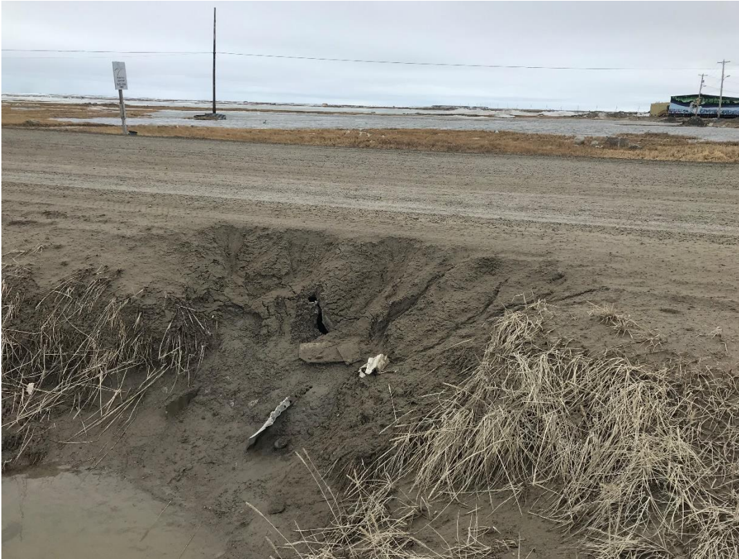
Figure 4: Extreme Example of Damaged/Blocked Culvert
