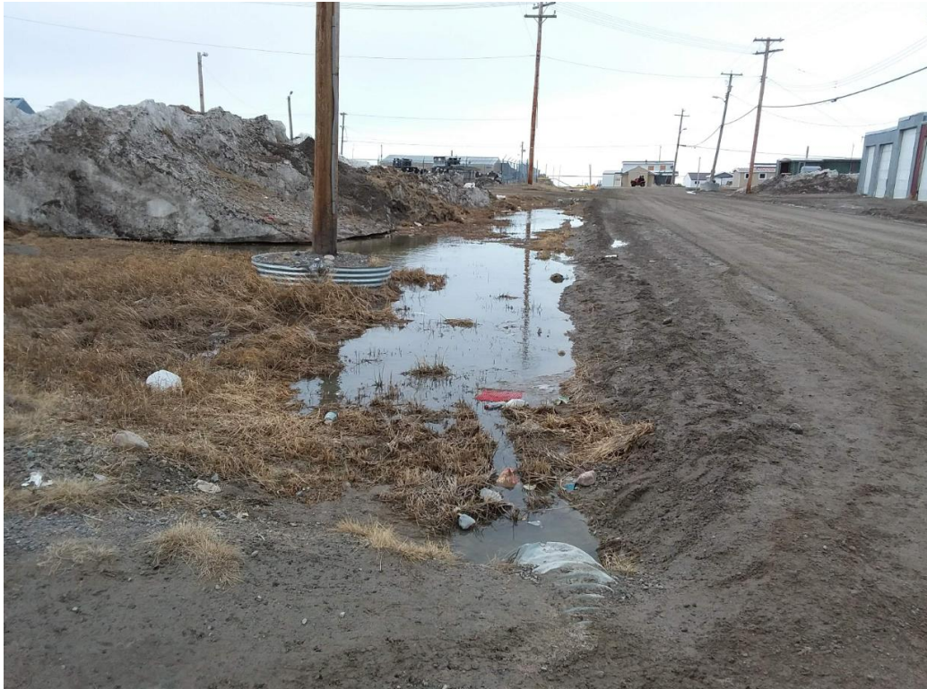
Figure 43: Looking north up 6 th street from end of culvert at Elders Centre
