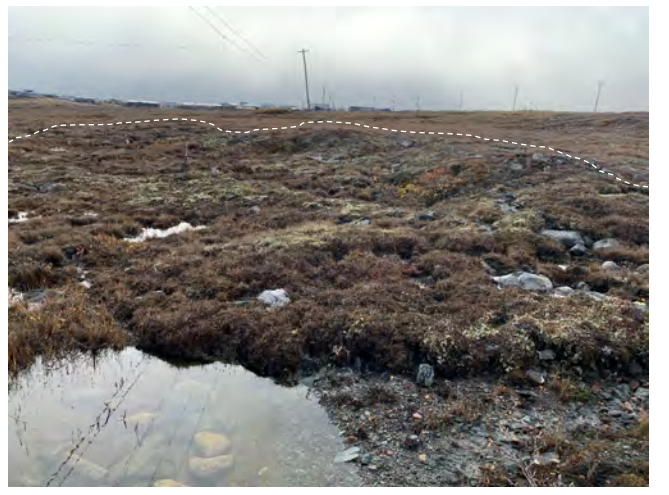
Photo 36: Potential signs of thaw degradation (tension cracks and ground subsidence) north of Block 10.
